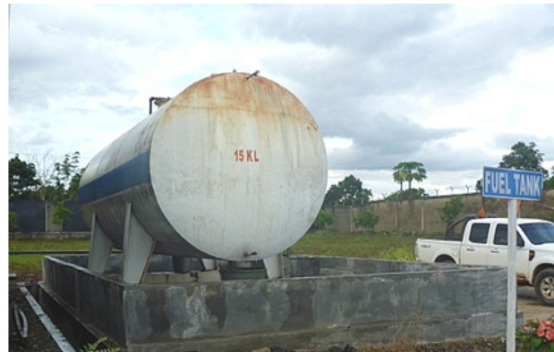
Sample of secondary containment of fuel tank.
