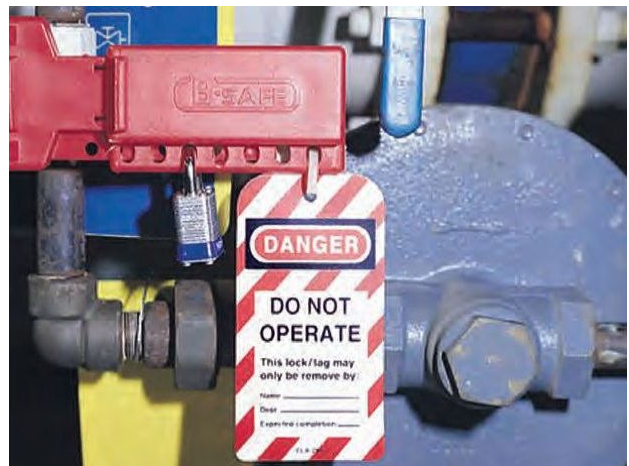
Figure 1. Lock Out/Tag Out (LOTO)
